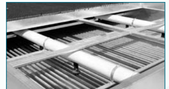
Drift Eliminators Removed for Coil Inspection
