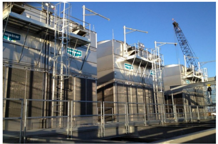
Figure 2 – Stainless steel cooling towers
