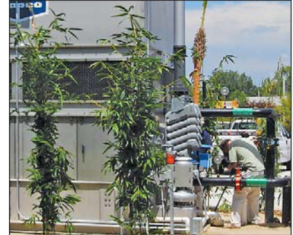
Closed Circuit Cooler Gainesville, FL USA
