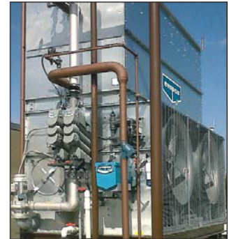
Evaporative Condenser Miami, FL USA
