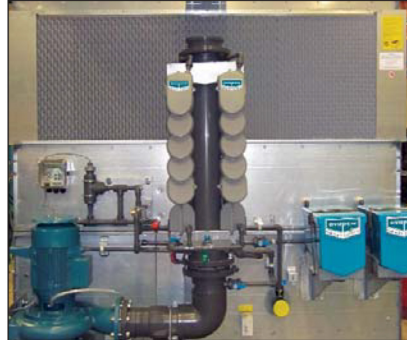
Closed Circuit Cooler Bruges, Belgium
