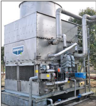
Closed Circuit Cooler Shanghai, China
